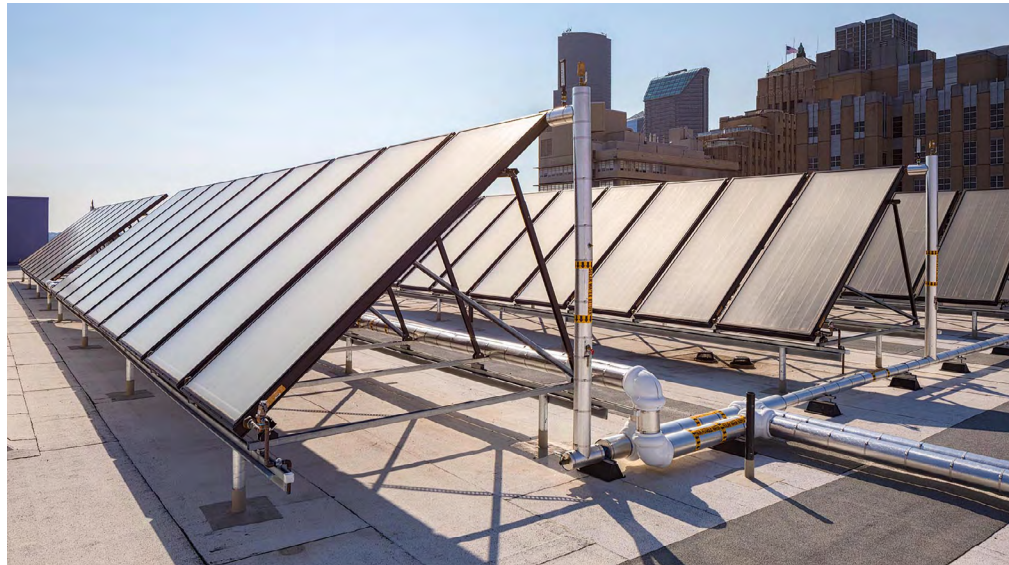
Solar array at Red Cedar Apartments, Yesler Terrace, Seattle
