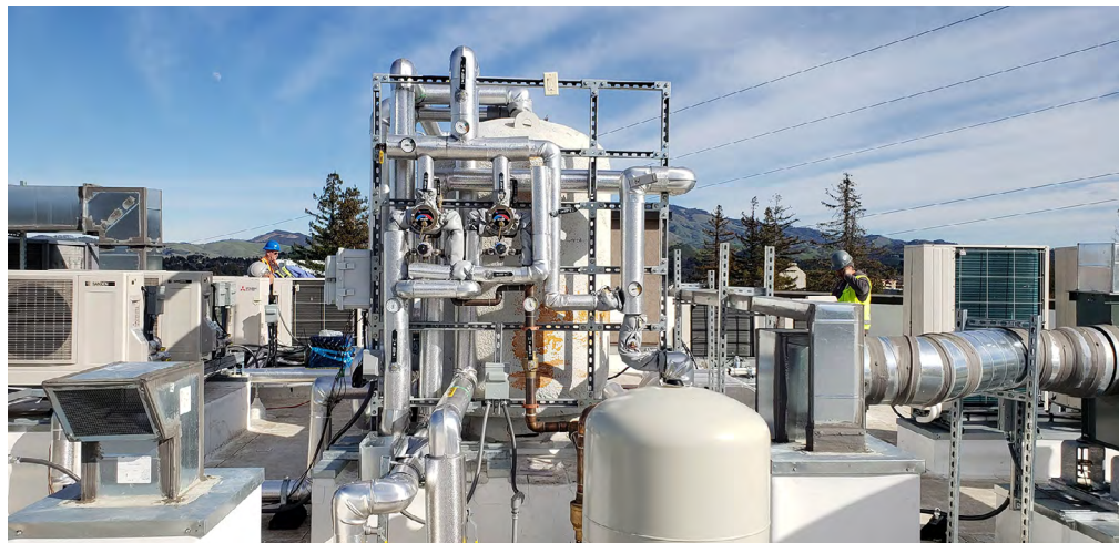
All-electric systems at St. Paul's Commons, Walnut Creek
